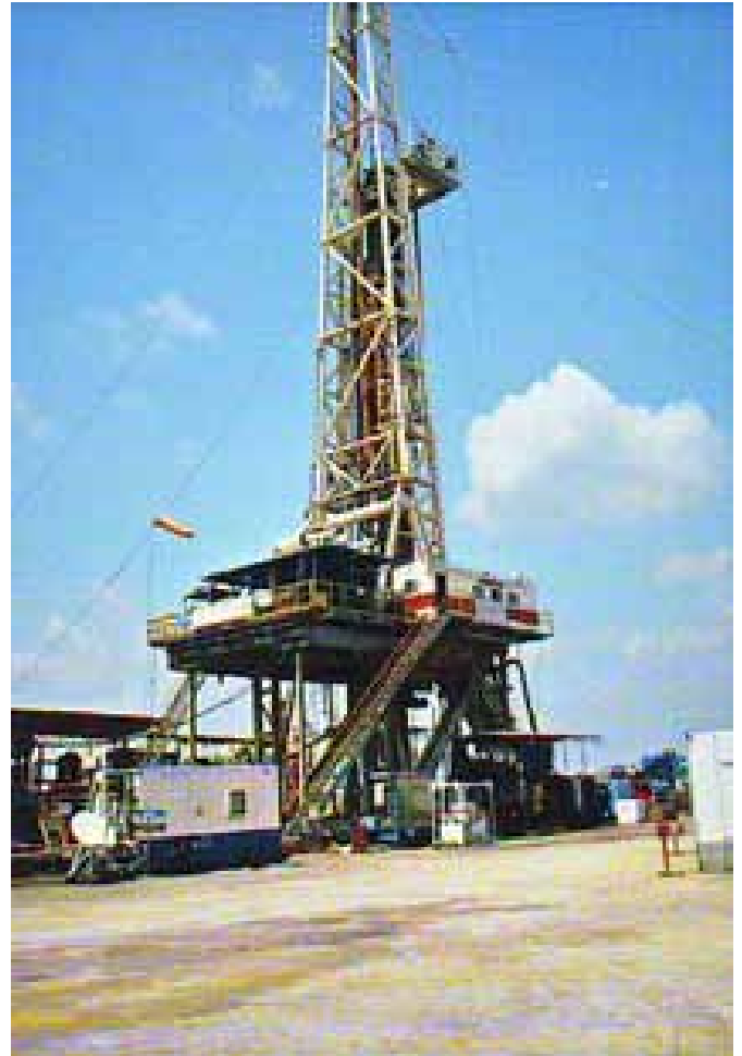
Figure 4. Active drilling at N. Kedungtuban #A, 15 km west of Cepu, with planned TD of nearly 3000 m.
